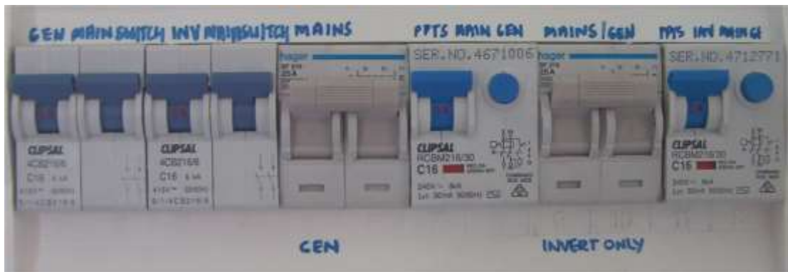
Figure 37 - Shore Power Set Up
