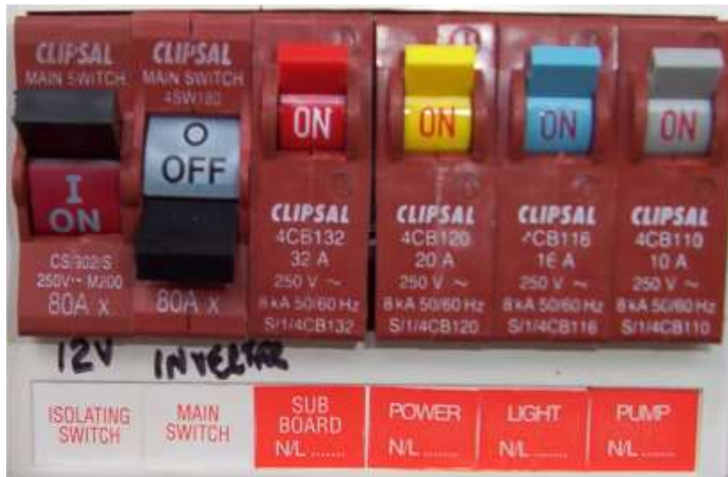
Figure 34 - D.C. Power On, No Inverter (Normal Setting)
