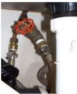
Figure 27 - Air Con. Water Tap
